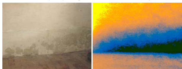
Figure 6. Moisture on a wall: visible (left) and IR images.
